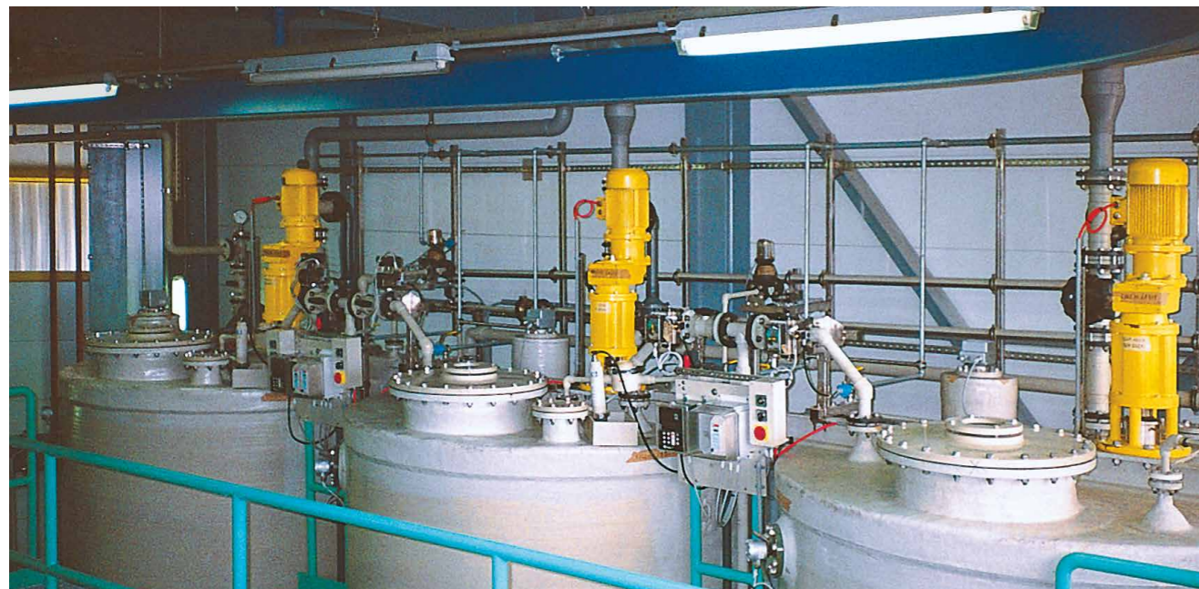
System to alkalinize influent stream with limestone.
