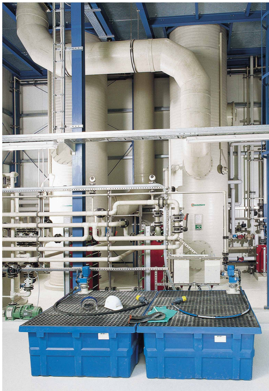
Ammonia recovery by air stripping.
