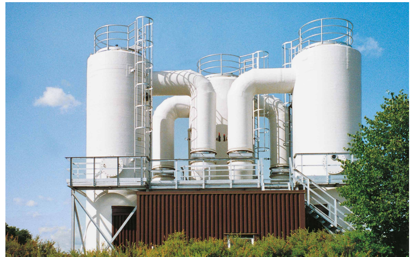
Air stripper for the treatment of reject effluent water at a wastewater treatment plant.
