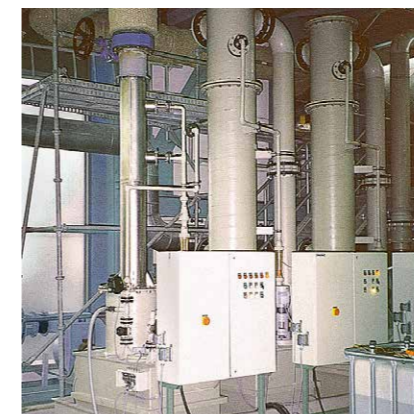
Bypass-plant for recovery of hydrochloric acid from flue gas.
