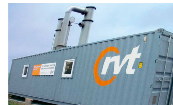
Equipment for injection of ammonia
