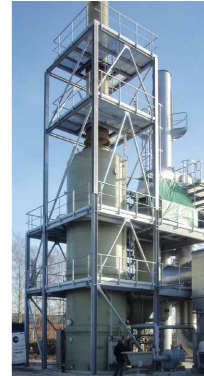
Single-stage waste gas scrubber behind a regenerative oxidizer of a chemical plant, 50,000 Nm 3 /h
