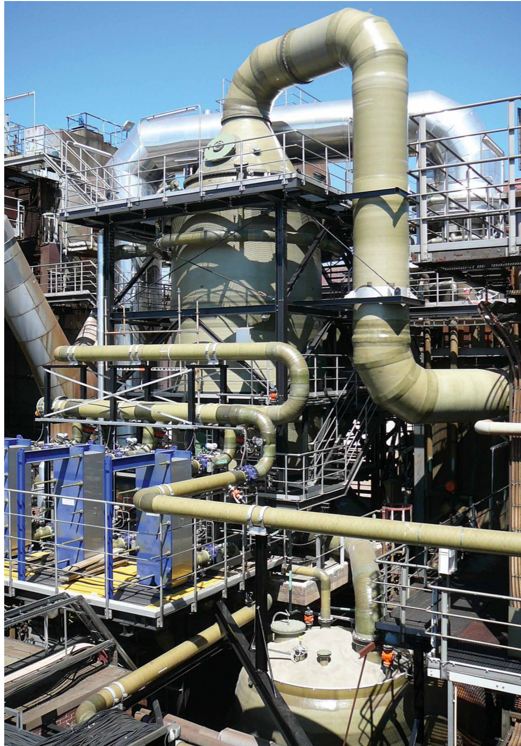
Cooling column with 3 heat exchangers in the foreground to utilize waste heat energy in a district heating system
