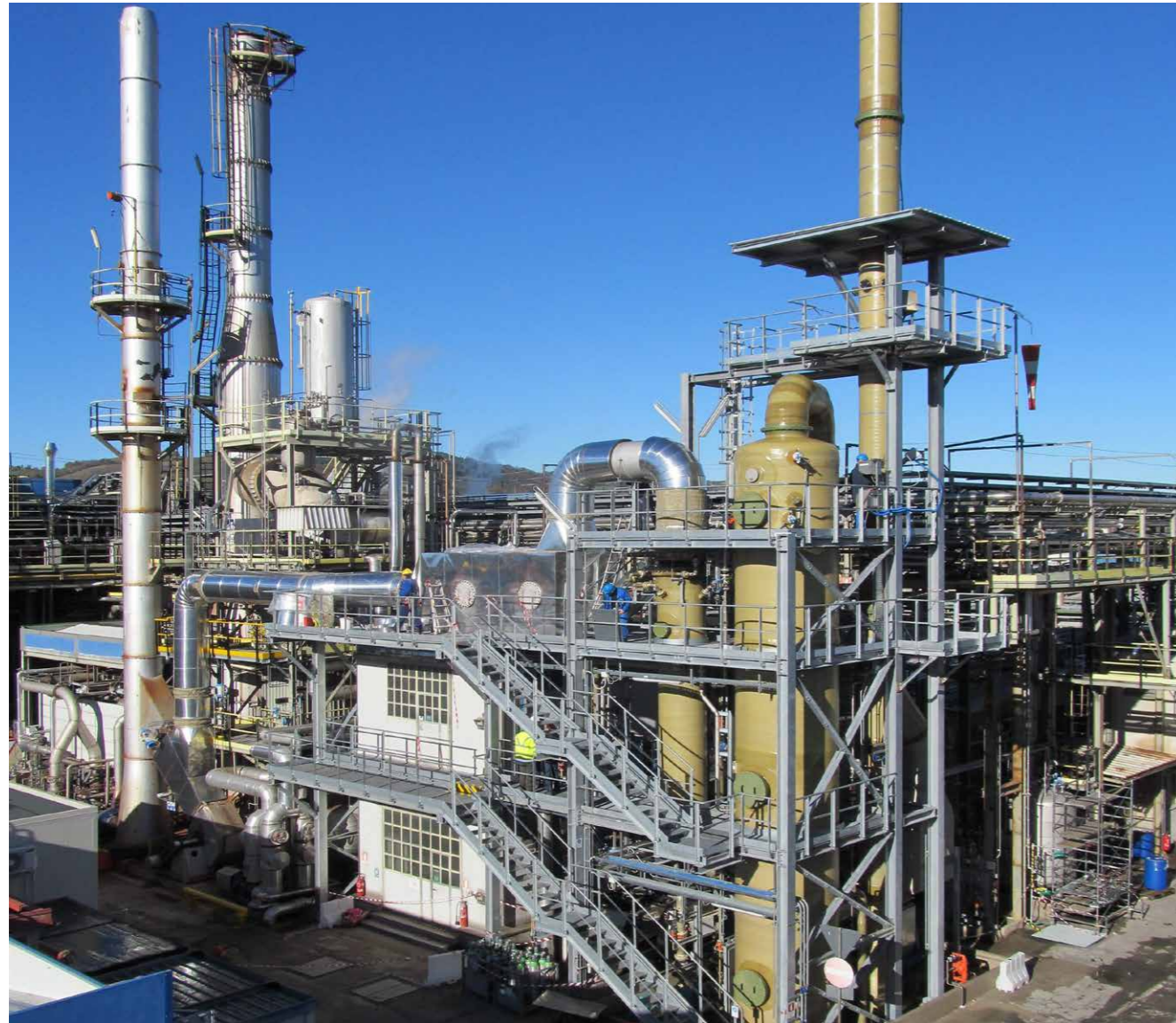
Waste gas cleaning plant with hot gas quench, SCR-reactor and multi-stage absorption, 20,000 Nm 3 /h
